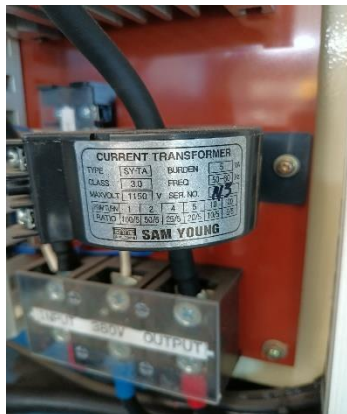
Gambar 5. Current Tranformer 50A
